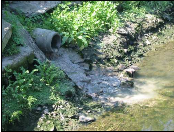
Discharge pipe at Clerkes Lane
