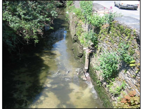
Discharge pipe at Clerkes Lane
